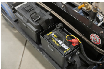
DUAL ON-BOARD 24V BATTERIES
